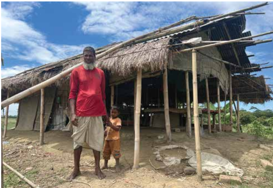
A man with his grandson standing in front of his dilapidated house in the middle of a haor (wetland) in Gowainghat, Sylhet on August 19, 200, just two months after the deadliest flood hit the region in decades.
